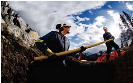
NATURAL GAS DISTRIBUTION $2,537M Rate Base
