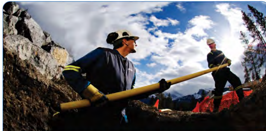
NATURAL GAS DISTRIBUTION $2,717M Rate Base
