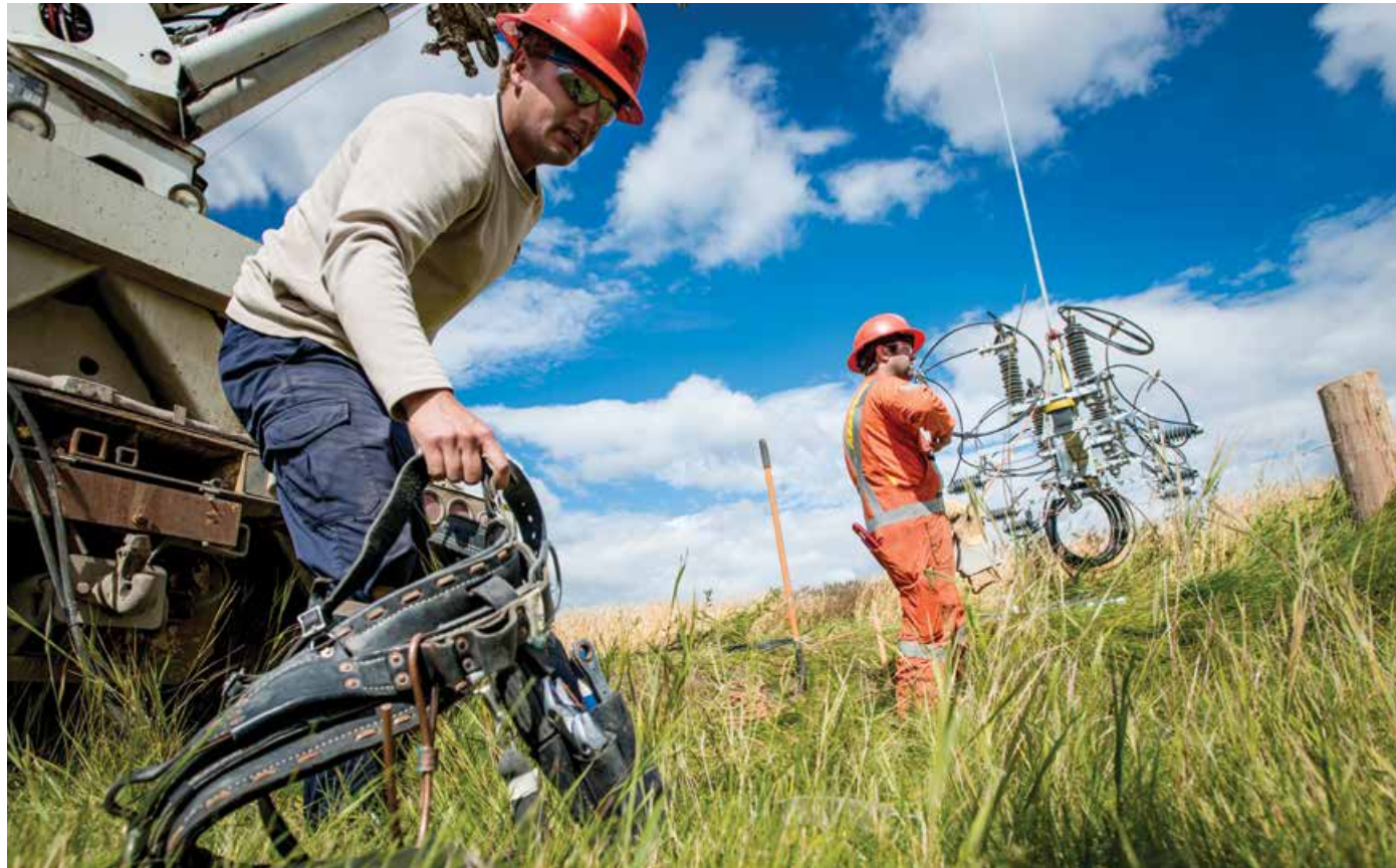
Safety is the first consideration in everything we do, and it's the responsibility of everyone on the work site - whether it's a powerline, pipeline, a lodge, a power plant, or the office.
