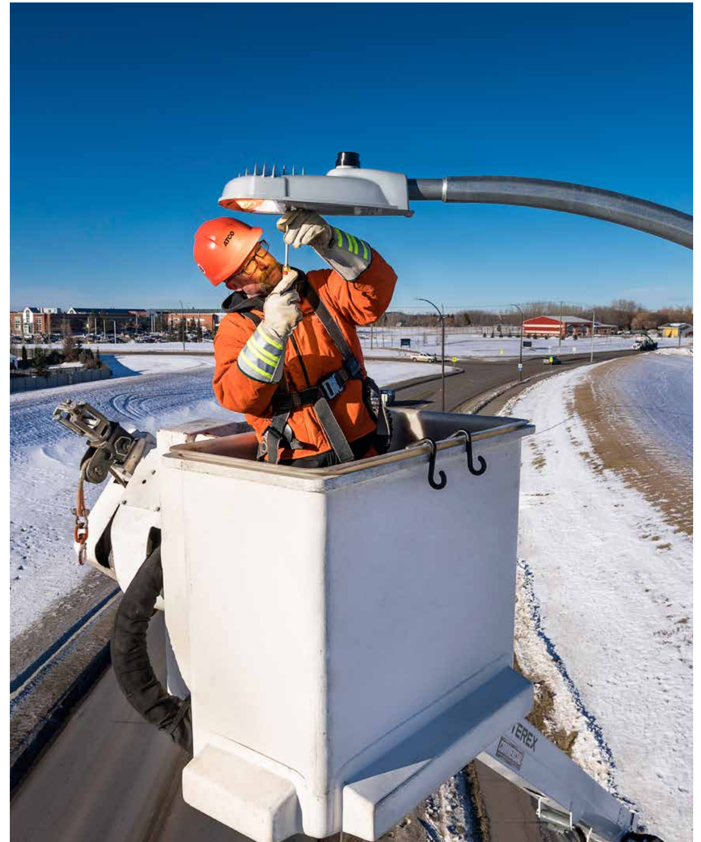
Our smart LED lighting solutions, like the one developed in Lloydminster, are helping our municipal customers conserve energy and reduce costs.
